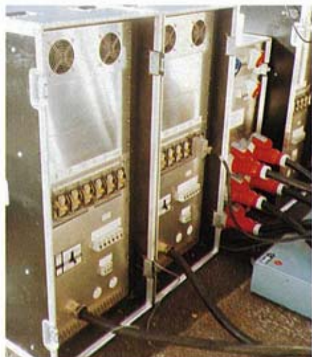
The dimmers, all multiplexed, were placed in five custom-built racks by Stage Electrics.
